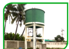
Common Overhead Tank
